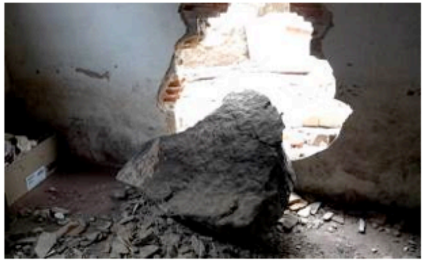
Figure 3 – Rock block invades residence Source: Colturato (2013).
