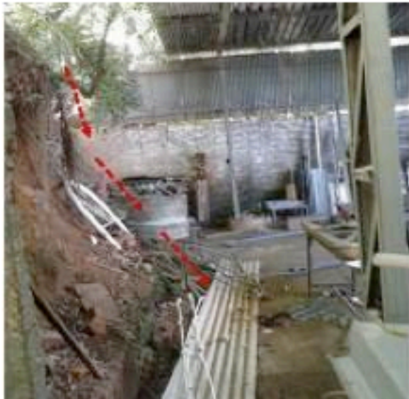
Figure 4 – Ground movement in the background of a commercial building. Source: Colturato (2013).
